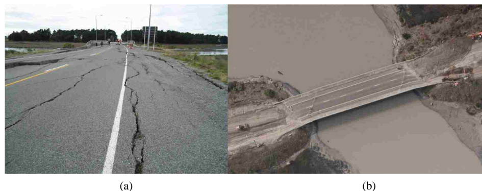
Figure 1.5: South Brighton Bridge after the Christchurch event. (a) Longitudinal lateral spreading cracks in western approach embankment (Cowan, 2011). (b) Aerial photo with visible lateral spreading cracks on river banks (LINZ, 2011).
