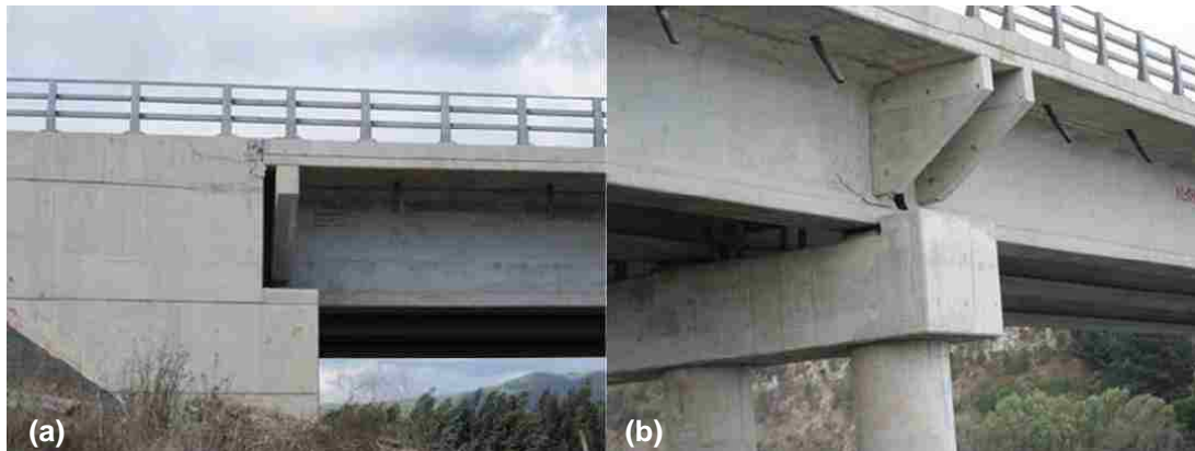
Figure 6.8: Minor structural damage caused by lateral spreading (GEER, 2010a). (a) Crushing of NE abutment. (b) Shearing of bridge girder above interior piers.
