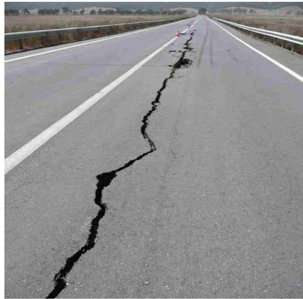
Figure 6.2: Longitudinal crack in northern approach to Puente Mataquito (GEER, 2010a).
