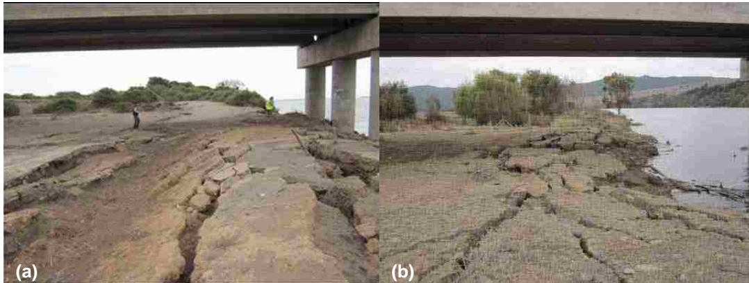
Figure 6.7: Surface manifestation of lateral spreading at Puente Mataquito. (a) Southwest approach (GEER, 2010a). (b) Northeast approach (MAE, 2010).
